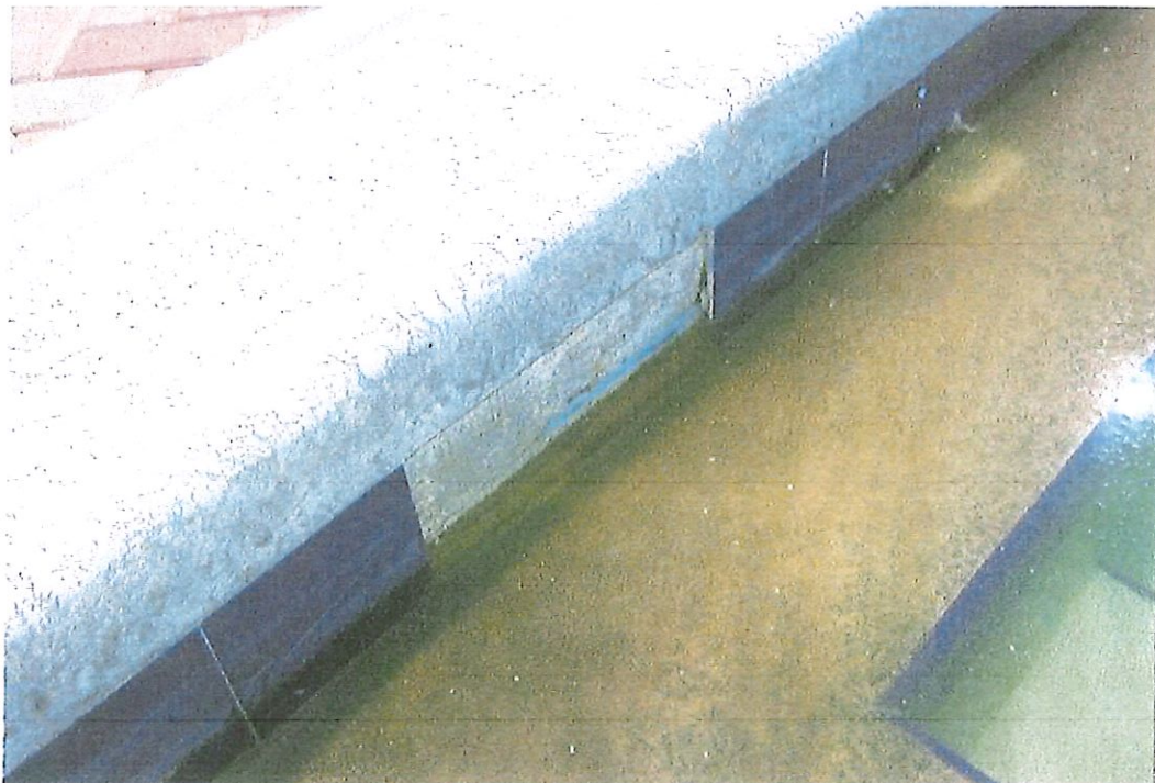
EXHIBIT 4. VIEW OF CRACKED WATERLINE TILES AND CRACKED POOL BEAM
